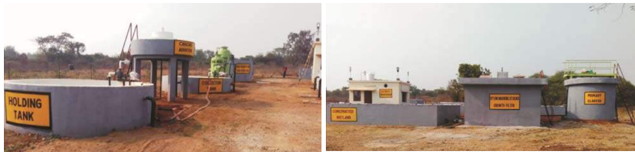
Ordnance Factory Ambajhari (OFAJ), Nagpur (Treatment Capacity: 100m 3 /day). The treatment system is under the commissioning phase.
