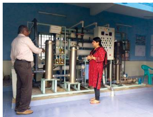
Water Treatment Facility at Mamsapuram, Virudhunagar District, Tamil Nadu
