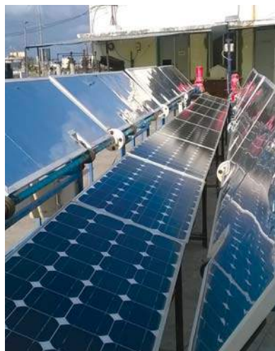
Community Scale PV powered desalination unit developed by CSMCRI, Bhavnagar
